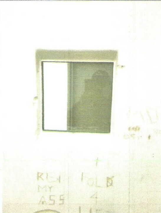
Repair gouges to padding surrounding cell door window.
