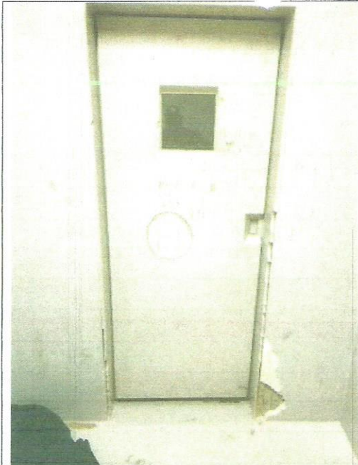
Repair Safety padding at Door jamb, and small gouges in safety padding. Repair gouges to padding surrounding cell door window.
